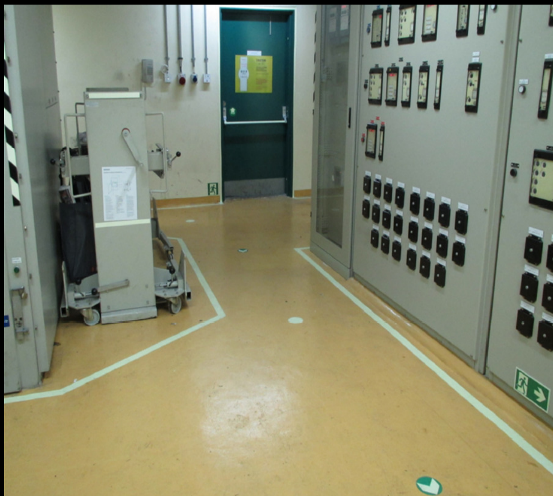
CEM, Macau, Power Plant HV Room
