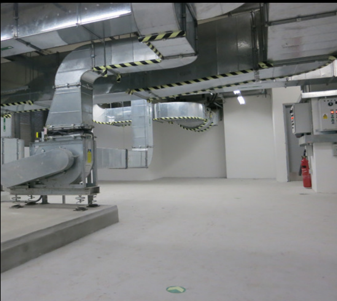
HSBC Data Centre, Plant Room
