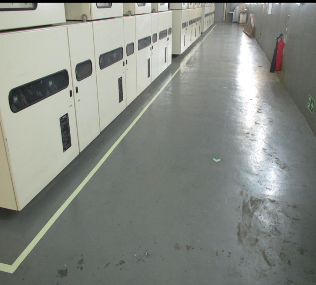
CEM, Macau, Power Substation
