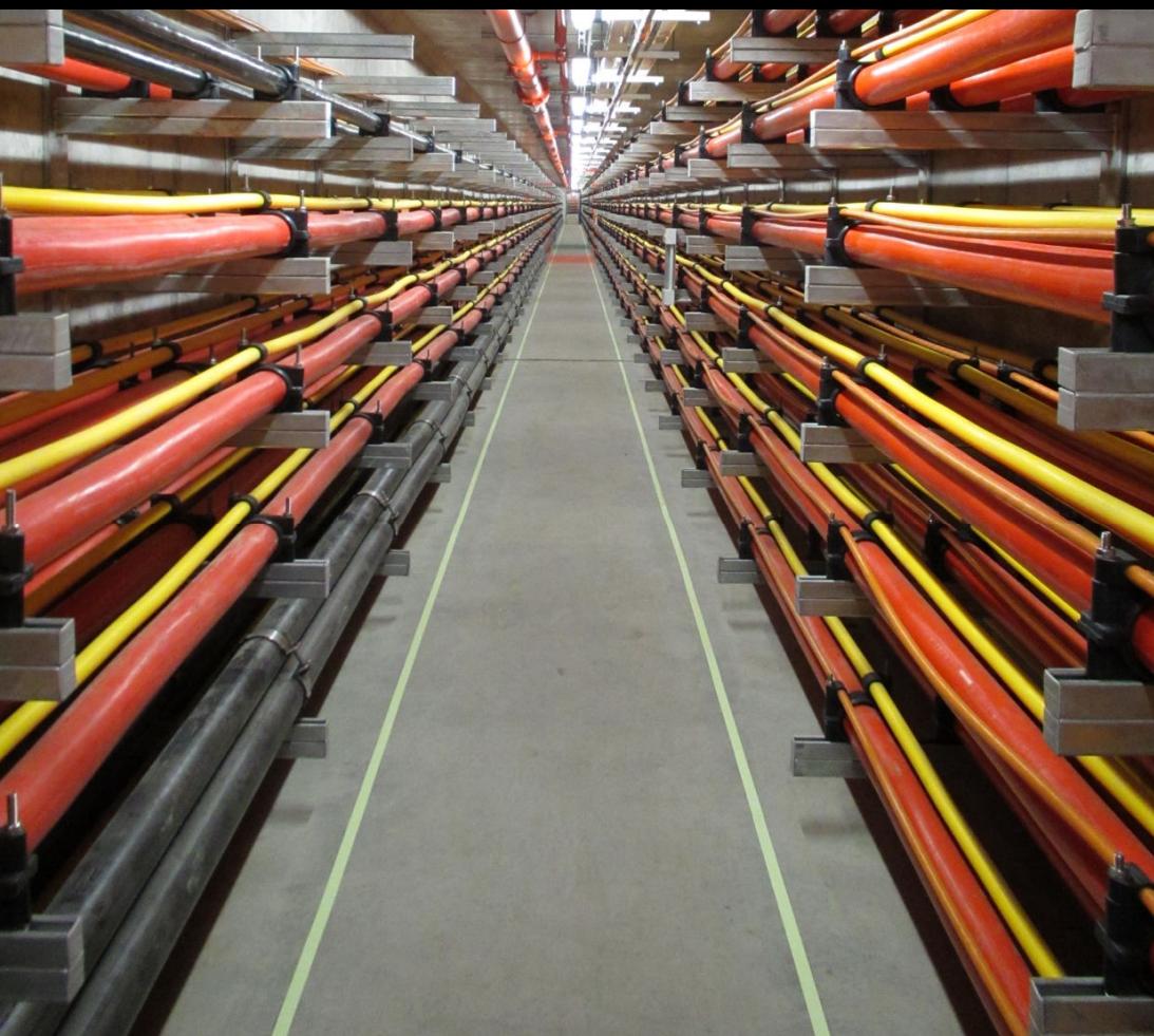
CLP, Cable Tunnel
