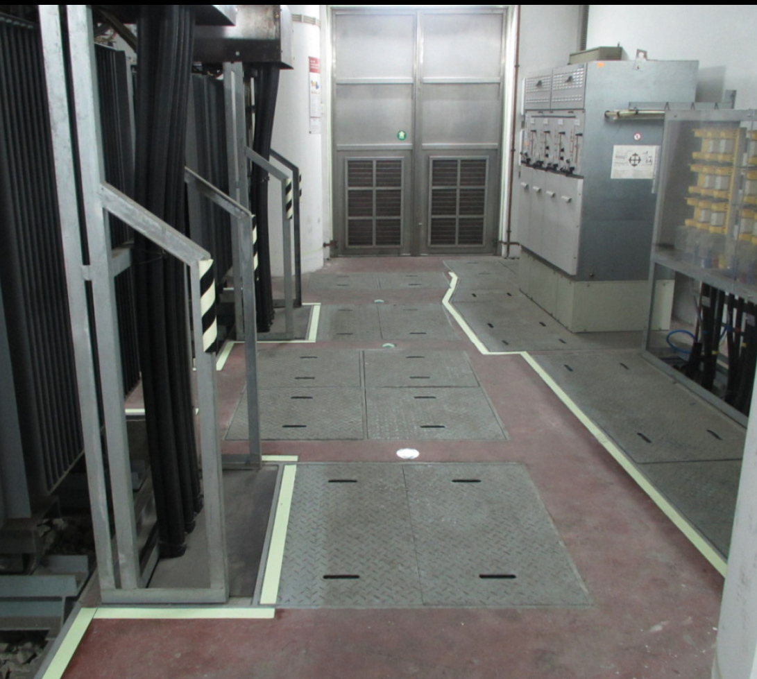
CEM, Macau, Power Transformer Room
