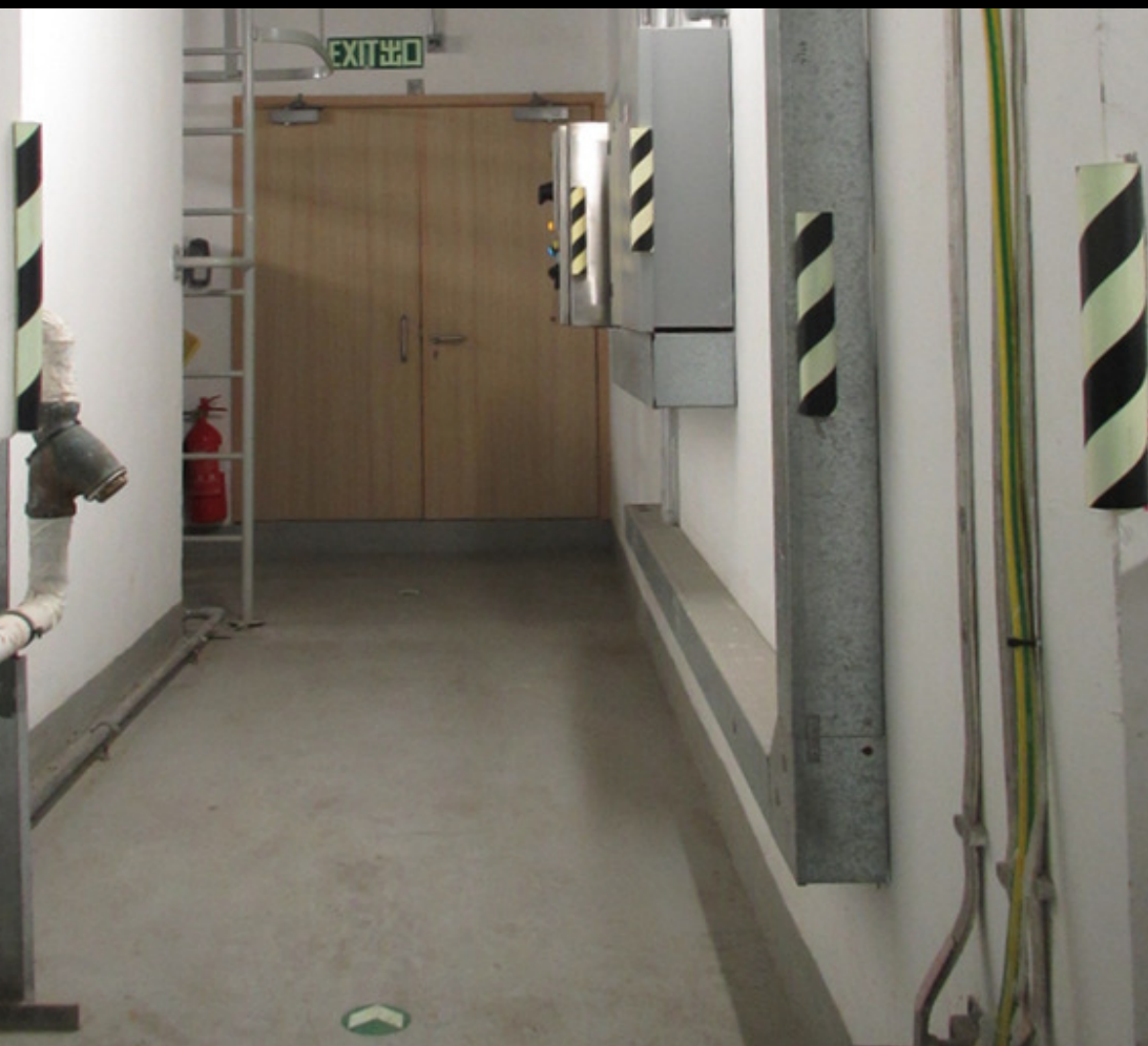
NTT Data Centre, Plant Room
