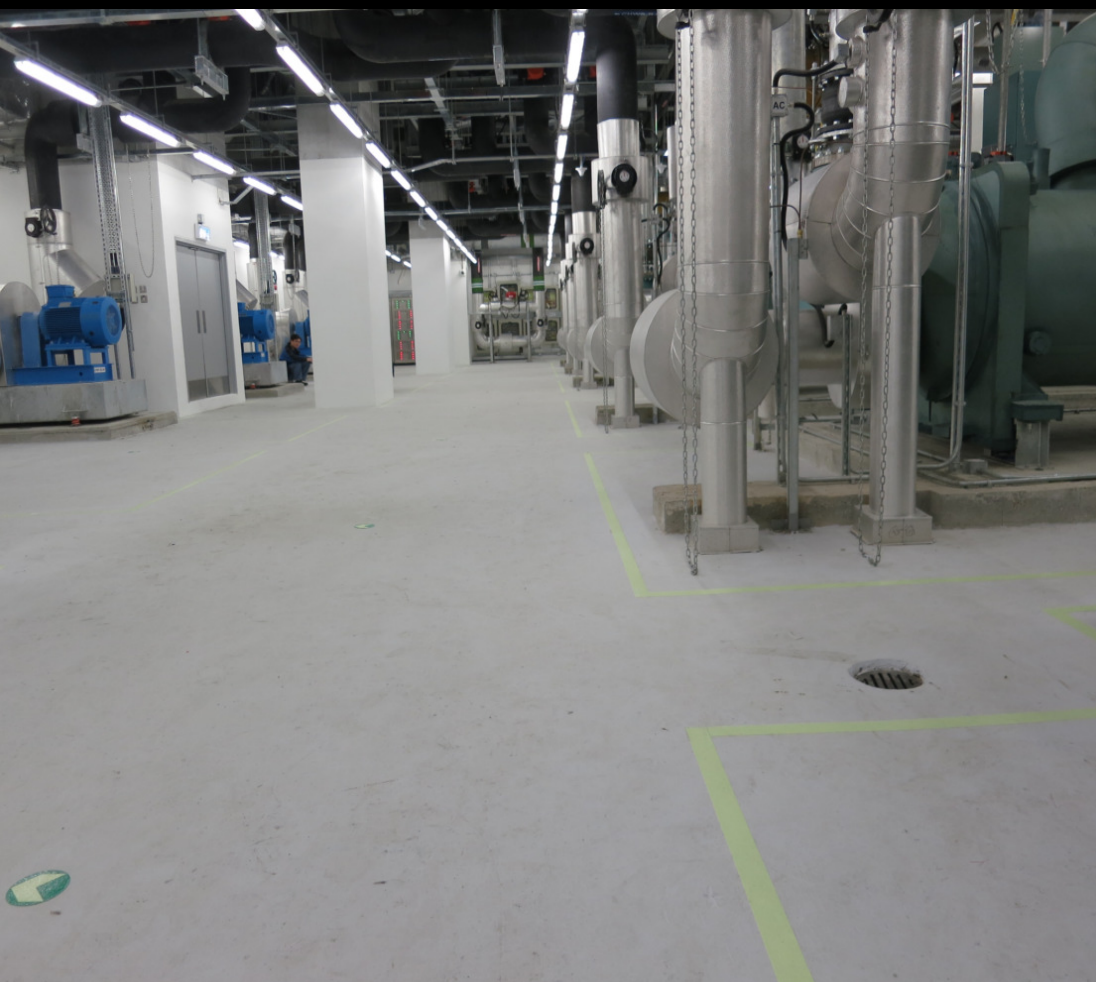
HSBC Data Centre, Plant Room
