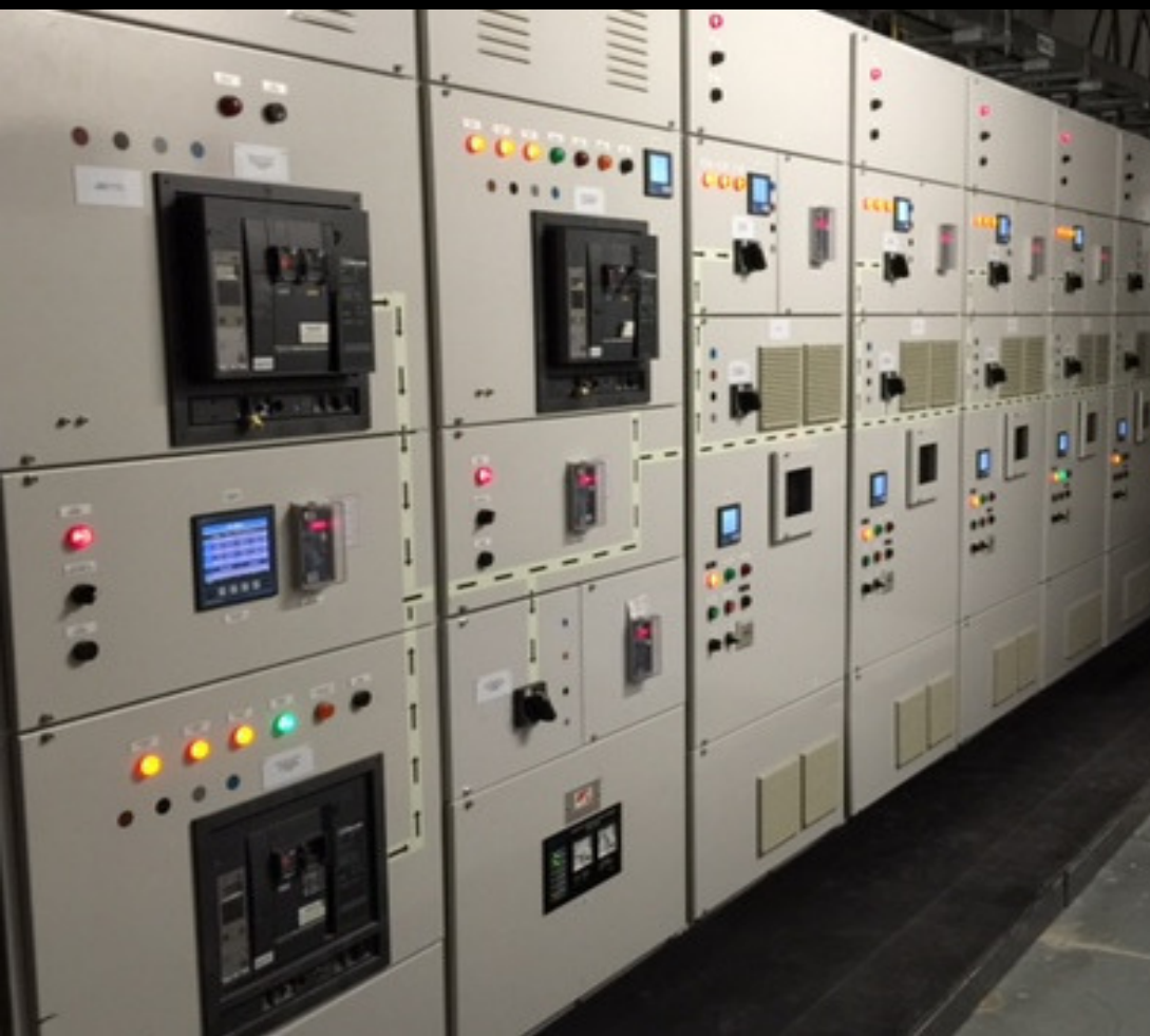
HSBC Data Centre, Plant Room
